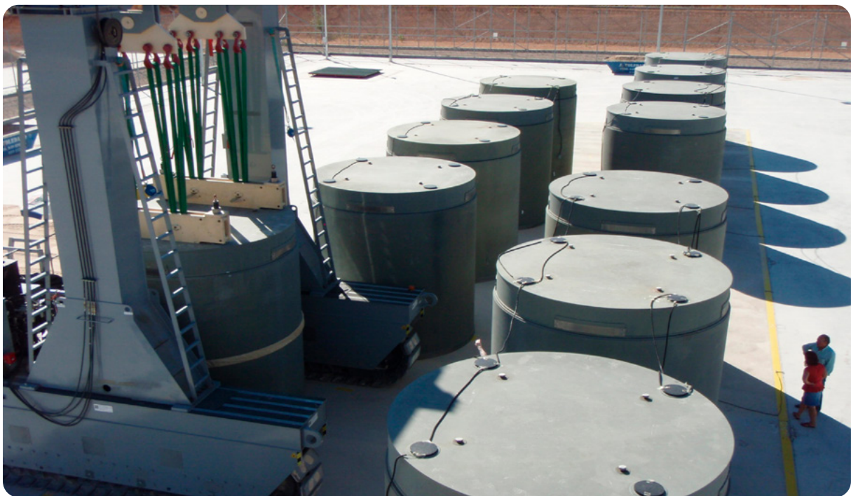
Figure 4-2: ITS casks at José Cabrera NPP
