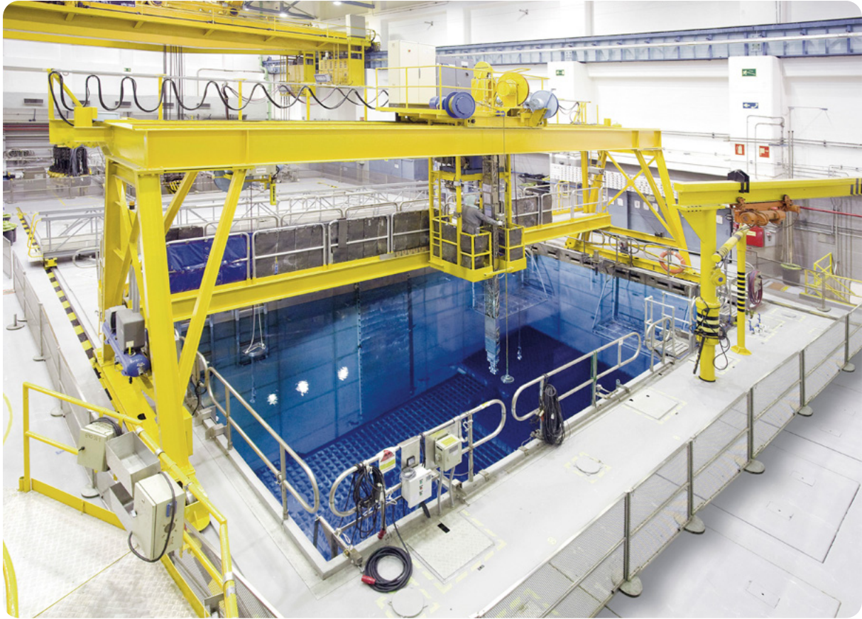
Figure 3-6: SF storage pool
